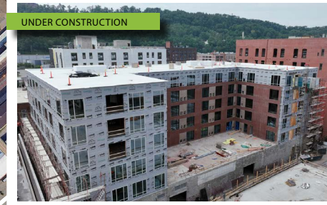
Conversion of a former Gateway Paints and Chemical Co. distribution center into a six-story, 105-unit apartment building
